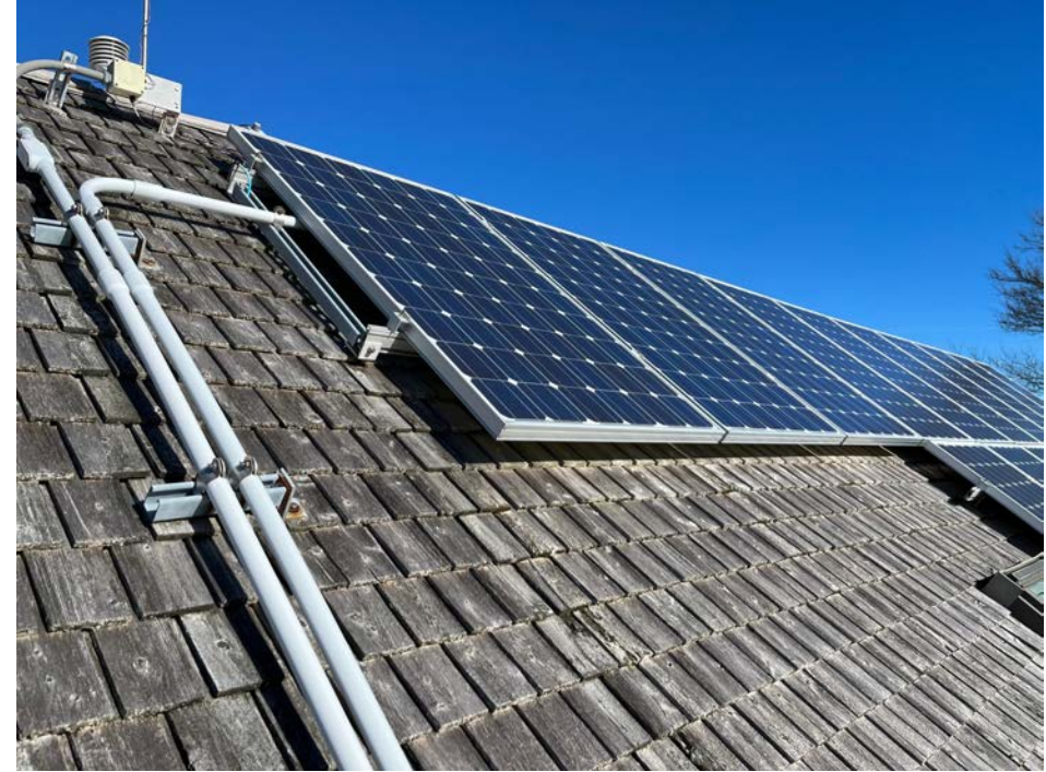
Distributed Solar PV
