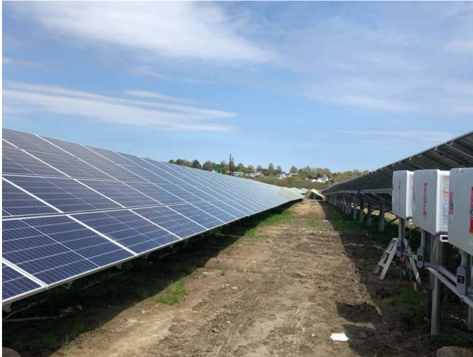
Utility-Scale Solar PV
