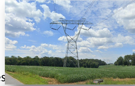
Example 500 kV structure
