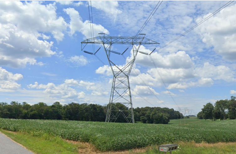
Example 500 kV structure
