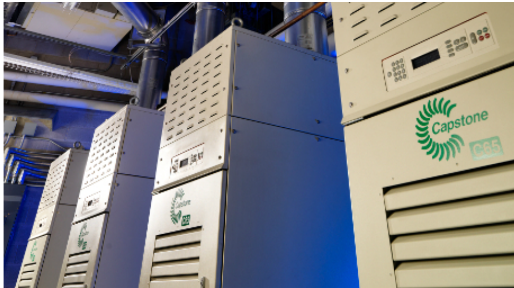
Huntington Center CHP system – Toledo, OH
